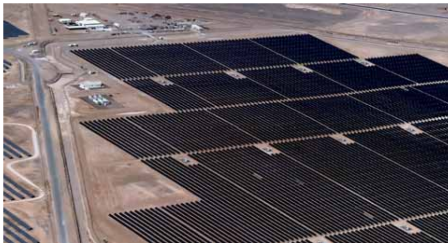
Credit: First Solar
