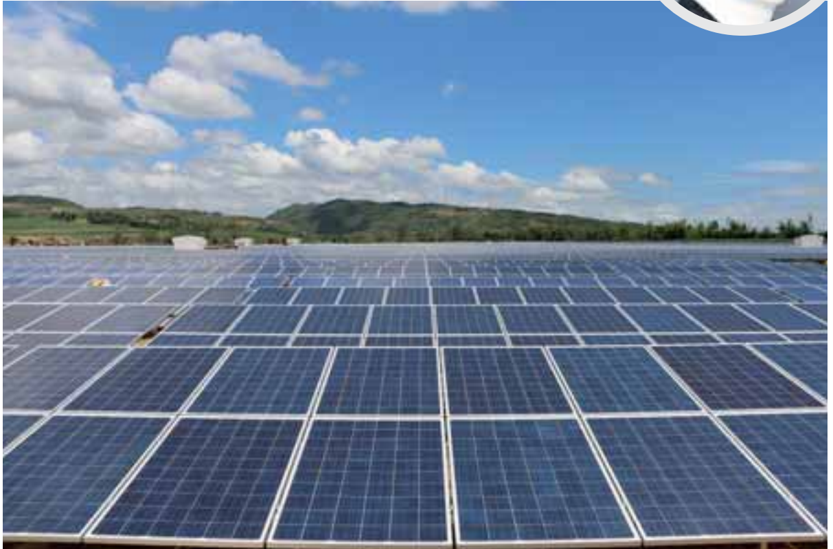
Credit: San Carlos Solar
